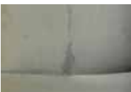
Indoor water damages
